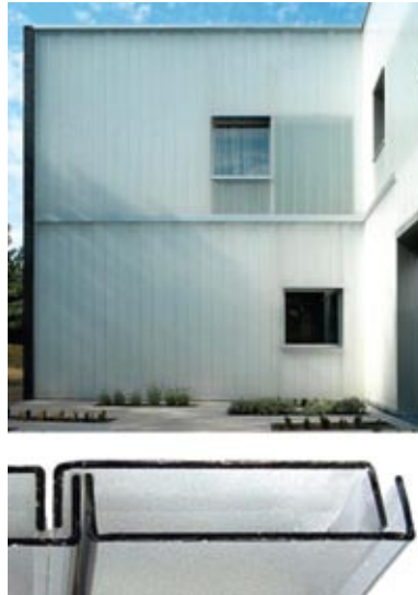
Figure 19: Library project Cladding System: Channel glass: Exterior side: Sandblasted, Interior side: 'carissimo' transparent. Top: Sample application; Bottom: Detail of channel glass connection.
